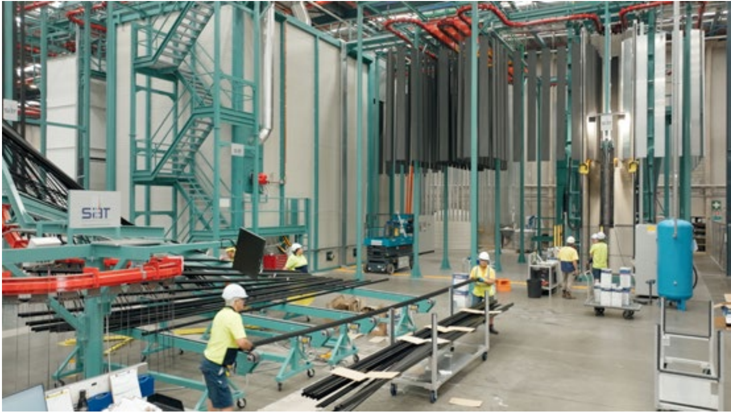
Capral Huntingwood Vertical Paint line commissioned in 2023
